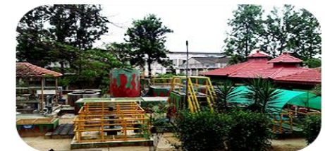
Effluent Treatment Plant Zero Discharge
